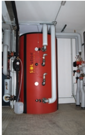
Buffer storage system
